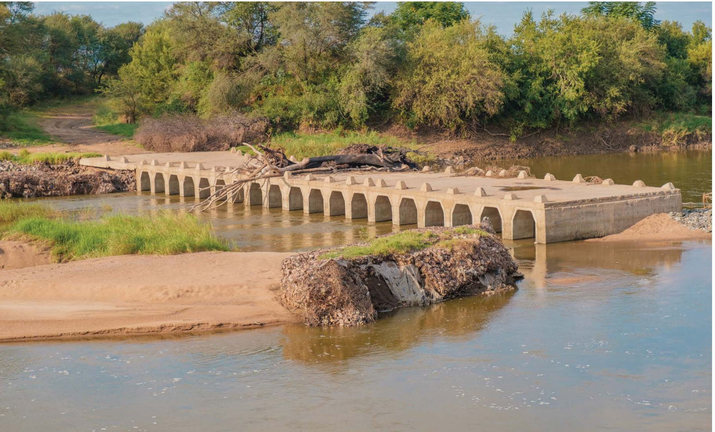
Washed out bridge on road D2357 in the Thabazimbi Local Municipality is due for restoration following the signing of strategic partnership between Roads Agency Limpopo and Northam Platinum Limited.
