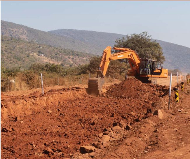
The construction project for road D3669, known as the Mavhunga access road, has commenced with considerable progress.
