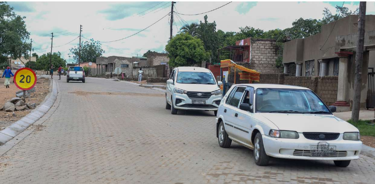
Construction in progress on Road D4424, a collaborative effort between Roads Agency Limpopo (RAL) and Palabora Mining Company (PMC). Some sections are now open to traffic.
