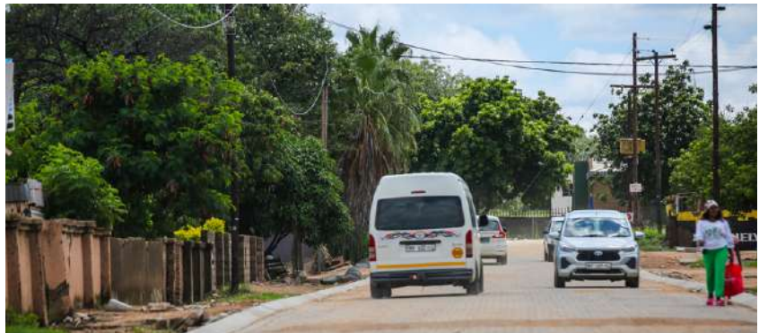
Some sections of road D4424 in Lulekani constructed as part of strategic partnership with Palabora Mining Company are now open to traffic affording motorists an immediate relief to the road's previous condition.
