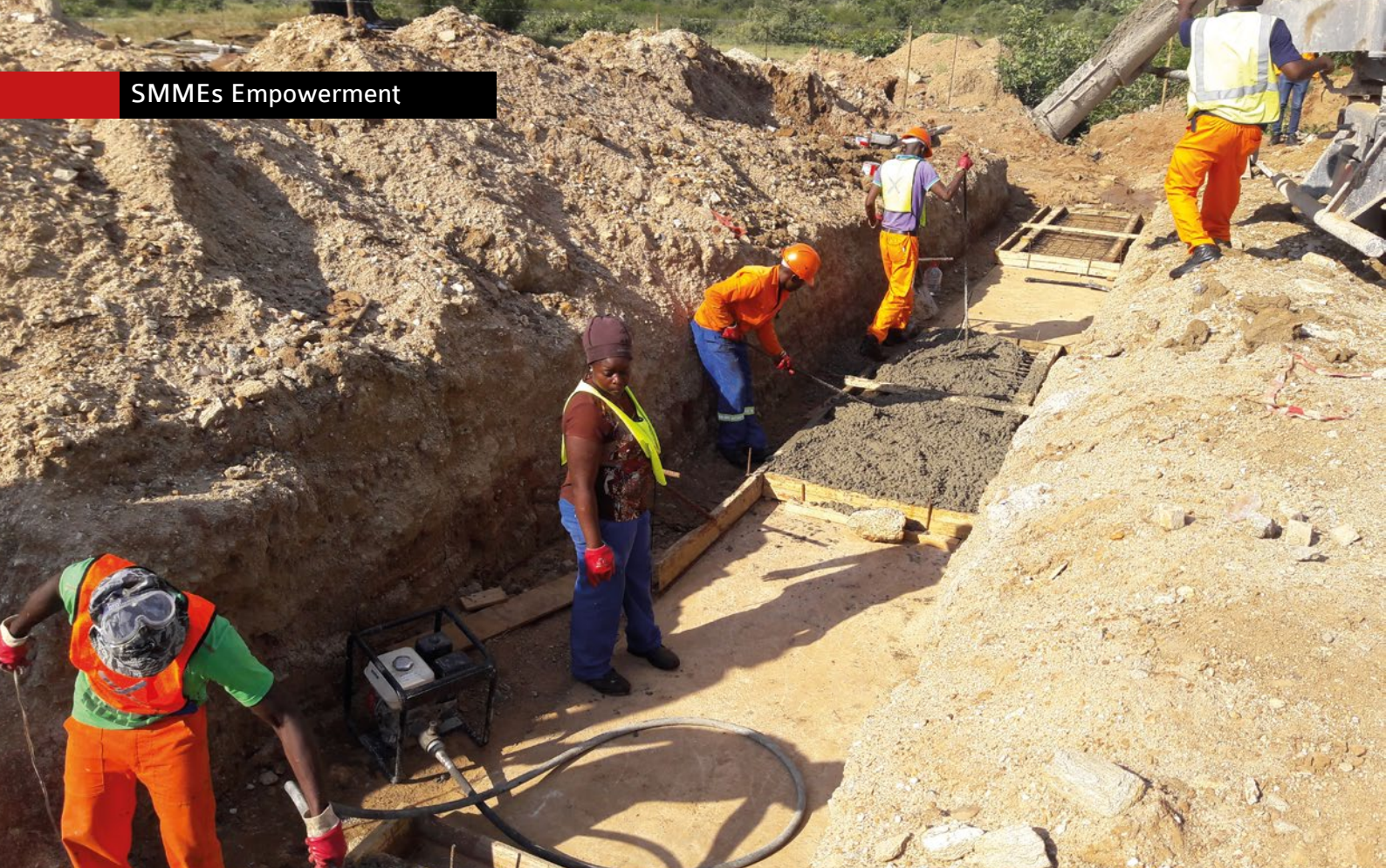
Mbanga Trading Enterprise, which was subcontracted to provide road earthworks, was one on the top performing SMMEs on the Ga-Ntata project for the reconstruction of two flood damaged bridges.
