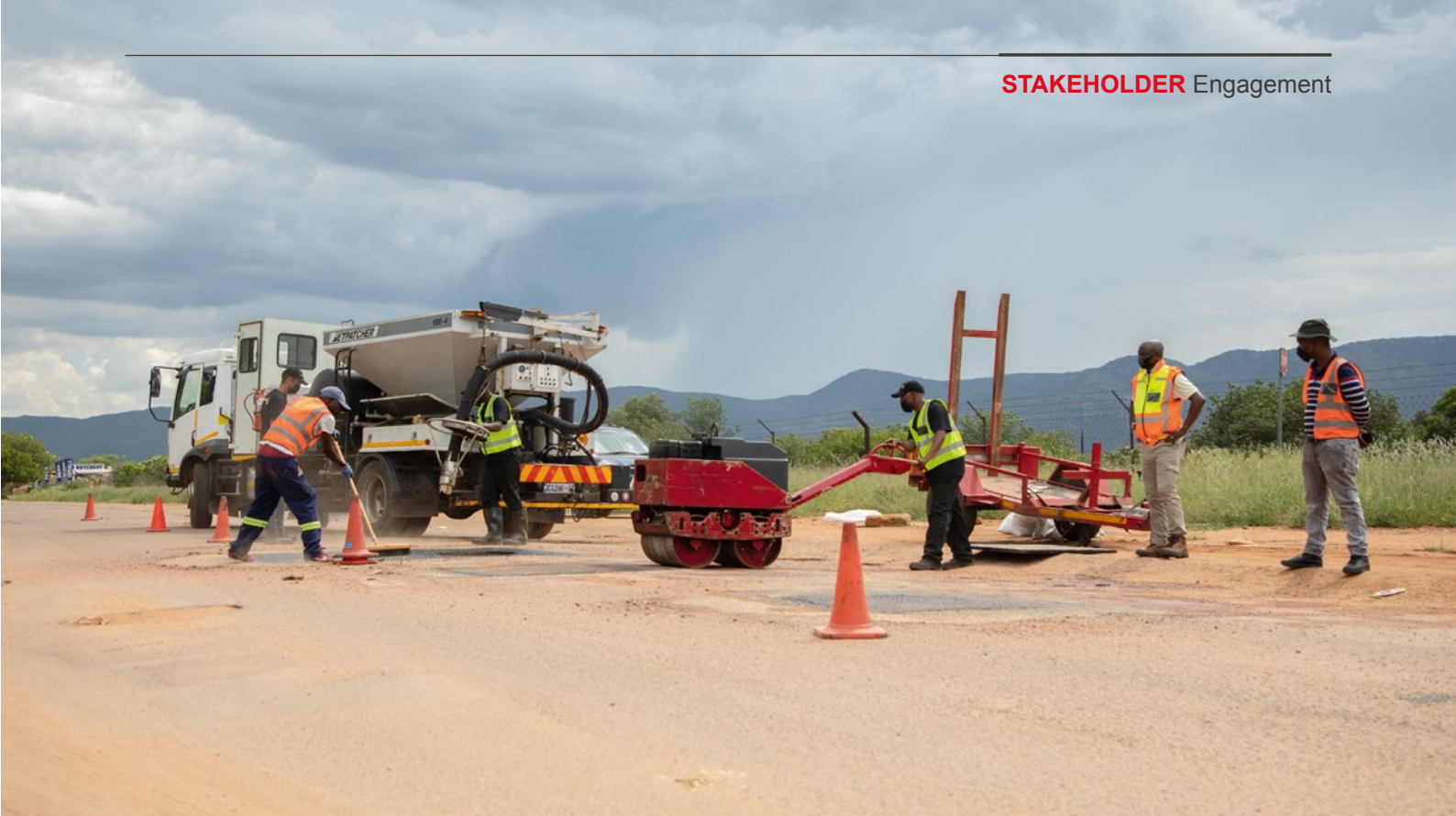
Gabriel Maluleke - RAL CEO (second from right) watches on while massive pothole patching goes in full swing in response to the dire road conditions in Mokopane town and the nearby areas in the Mogalakwena Local Municipality.
