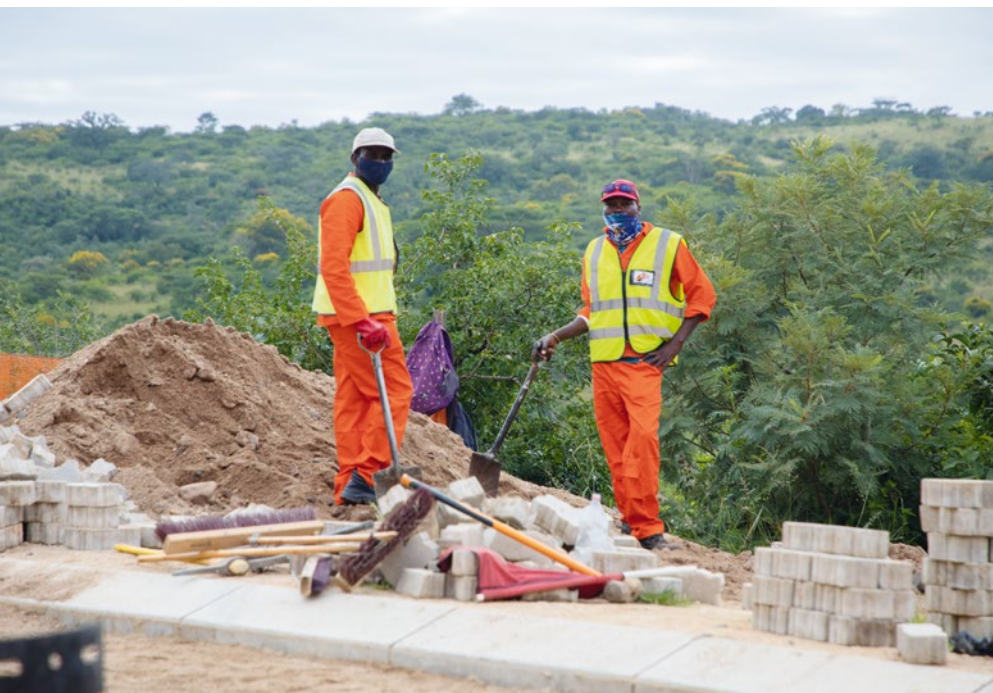
Some of the community members from the Mopani and Capricorn districts who were employed during block paving of road D3232 at Thakgalane village.
