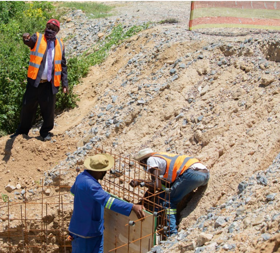
As one of the SMMEs beneficiaries, Solomon Ramashia from Ga-Raphahlelo village and Director of Tally Brand (Pty) Ltd is contracted on the project since September 2021 to build V-drains along road D15.
