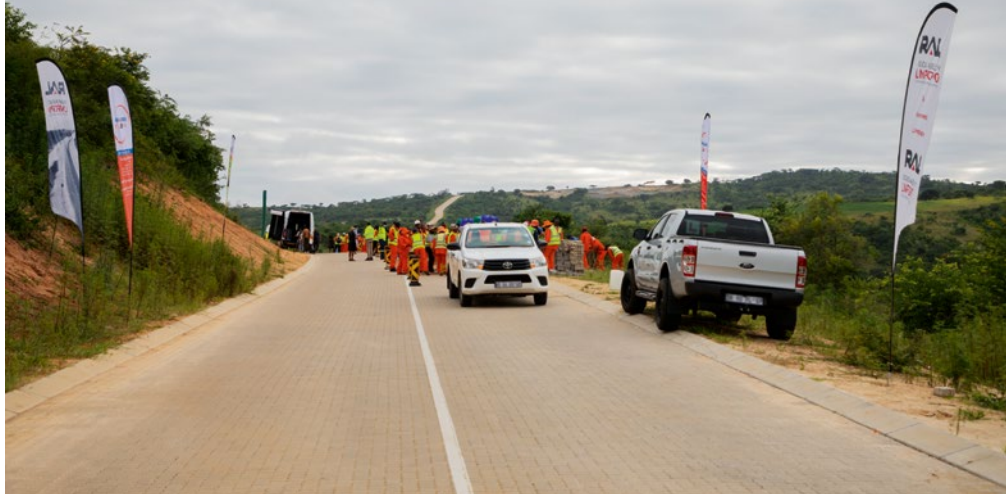
Prior to the Presidential Oversight Visit, part of Road D3232 literally constructed by local labourers with pave bricks at a glance.
