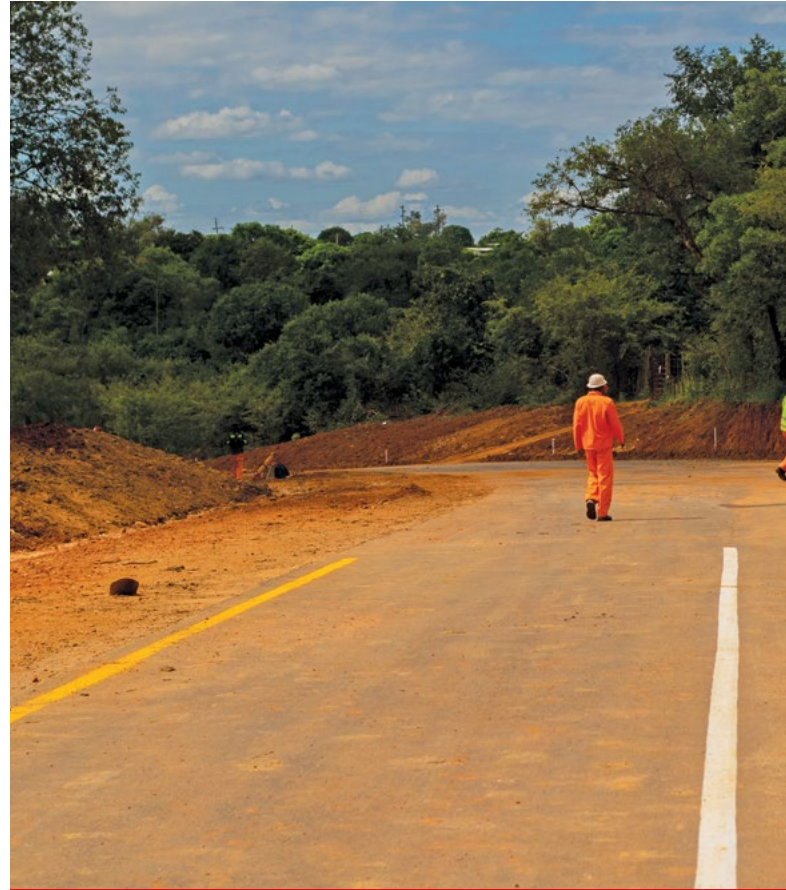
Phase one of RAL-led road D3248 project in N’wamitwa provided job opportunities to 51 local labourers, uplifted the socio-economic status.
