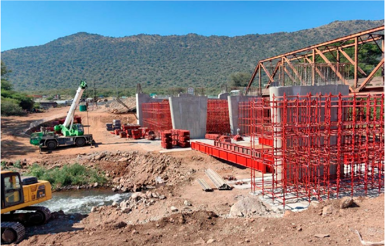
RAL STRATEGIC PARTNERSHIP APPROACH YIELD TANGABLE RESULTS: The Steel Bridge project on road D2219 in Ga-Malekana, a joint effort between RAL and eight mining companies operating in Sekhukhune. The project is progressing smoothly, currently at a 45% implementation stage.
