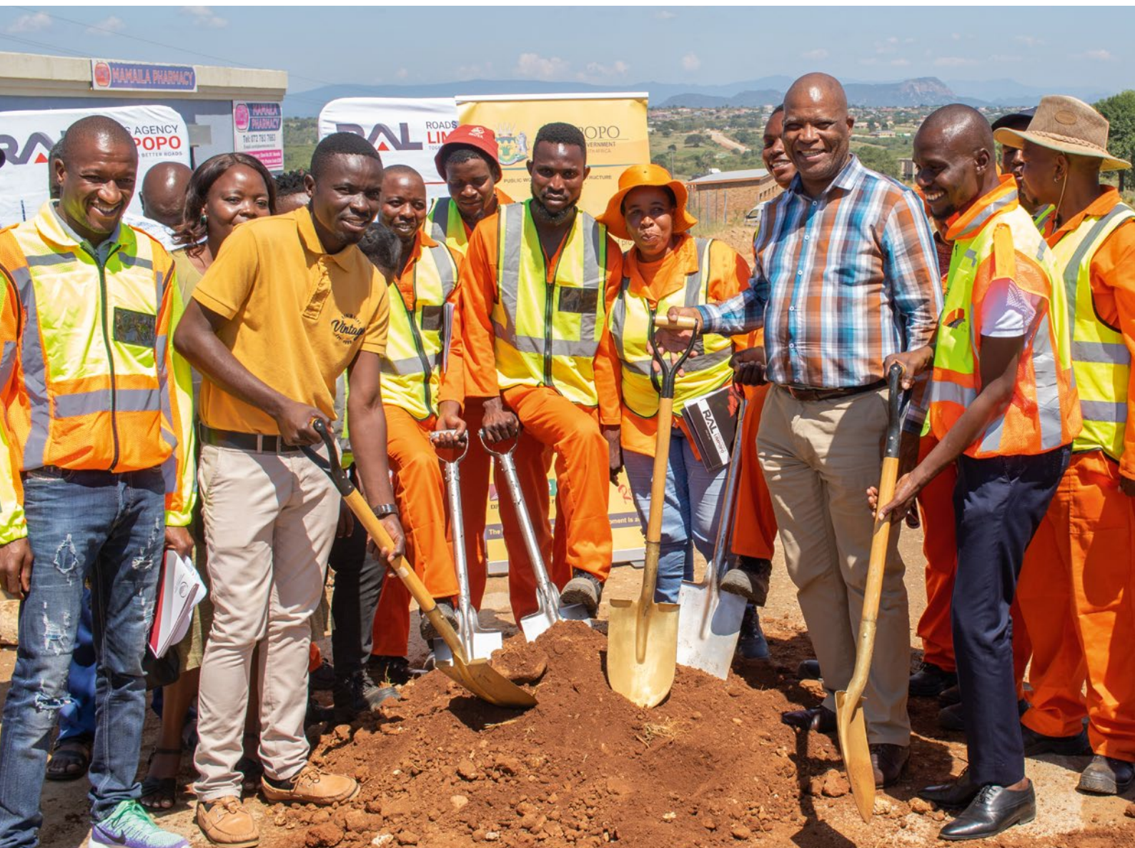
MEC for LDPWRI, Dr Namane Dickson Masemola joined by local labourers and leaders at the launch of one of the preventative maintenance road projects at Roerfontein, Mamaila Kolobetona Village within the Mopani District.
