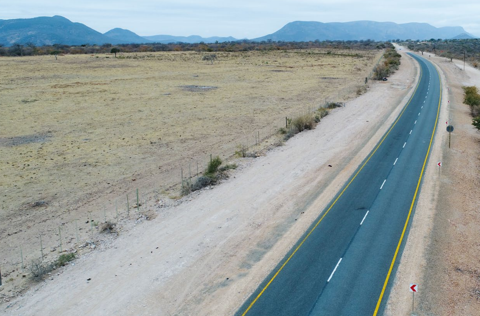
The recent rehabilitation and upgrade of provincial road D3671 towards the village of Musekwa in the Makhado Local Municipality of Vhembe District was built on the blood, sweat and tears of community members from various villages in the area.
